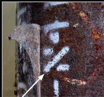
API 5L piping
