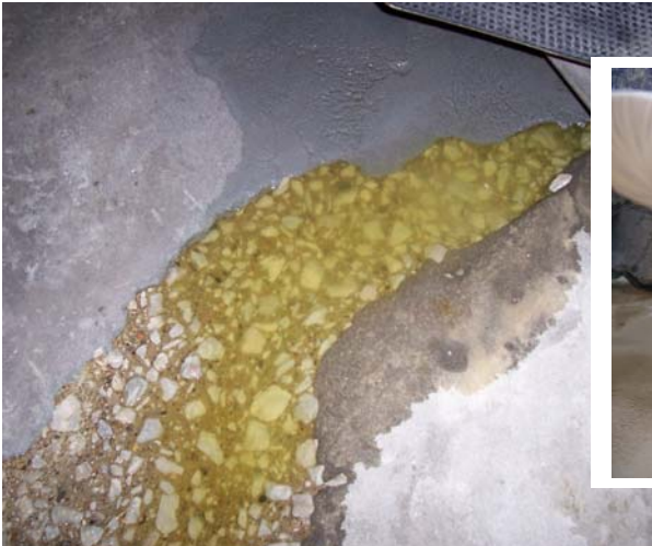
Citric Acid attacking the previous coating and concrete
